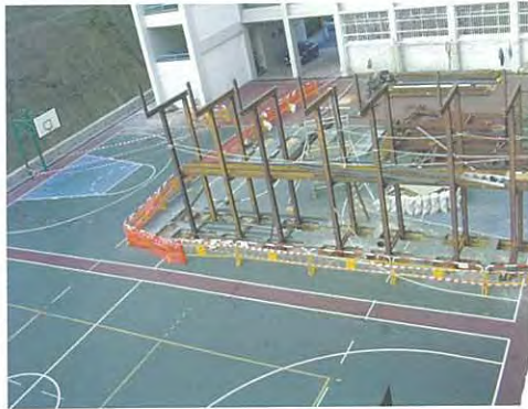
Building materials were delivered to the school and workers were preparing for the construction of scaffolding.
