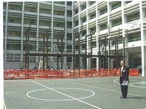
Workers were busy building the scaffolding on the fringe of the construction site.
