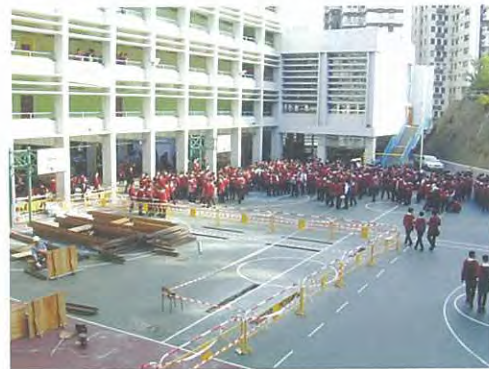
This picture shows the last assembly before the commencement of the construction project.
